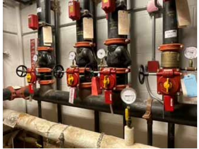
26 - FIRE SUPPRESSION SYSTEM
