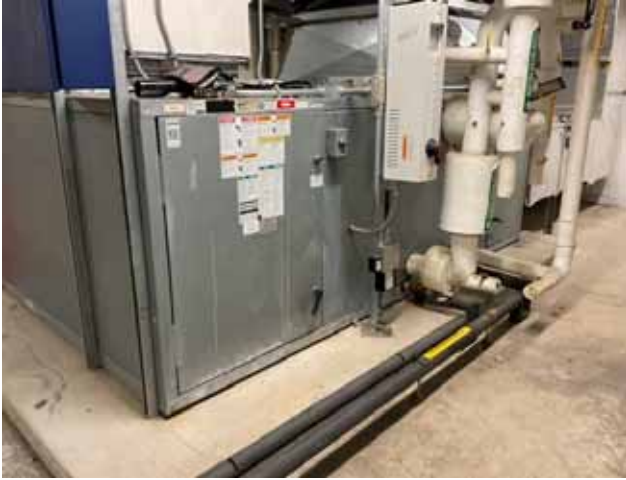
25 - AIR HANDLING UNIT
