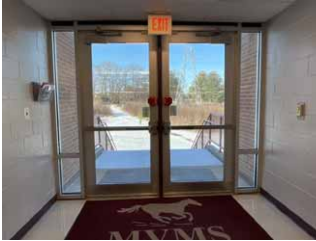
31 - FIRE ALARM SYSTEM
